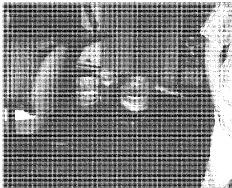
Leaking roof at Atlanta Center
