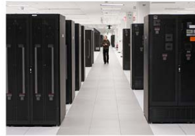
IBM Data Center, Present
